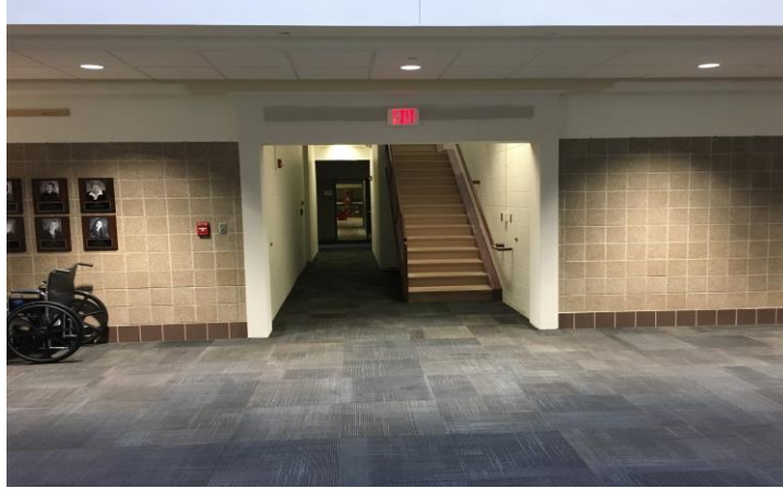
Across from Auditorium – removed single door and opened stairwell to Workforce Development lab
